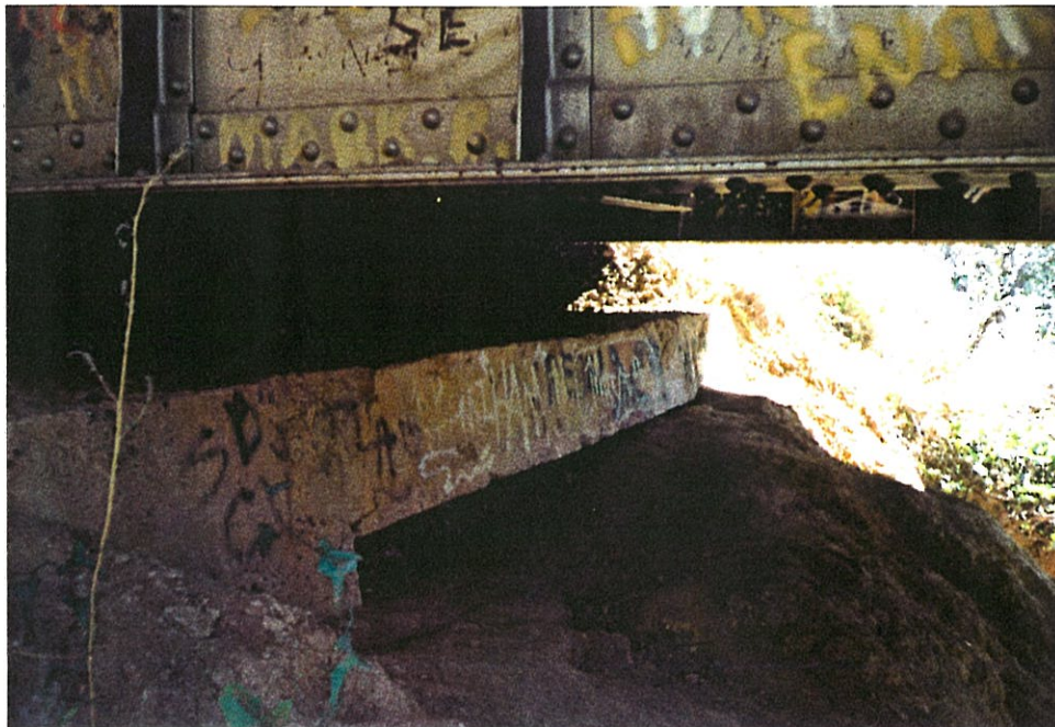
Photo 10: View of erosion at east abutment.
